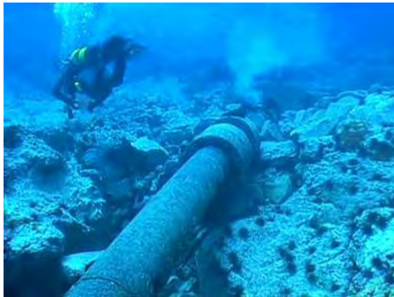
Fig. 4 Leak due to pipe breaking
