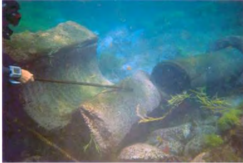
Fig. 3 Broken pipe caused by a mooring block during a tempest
